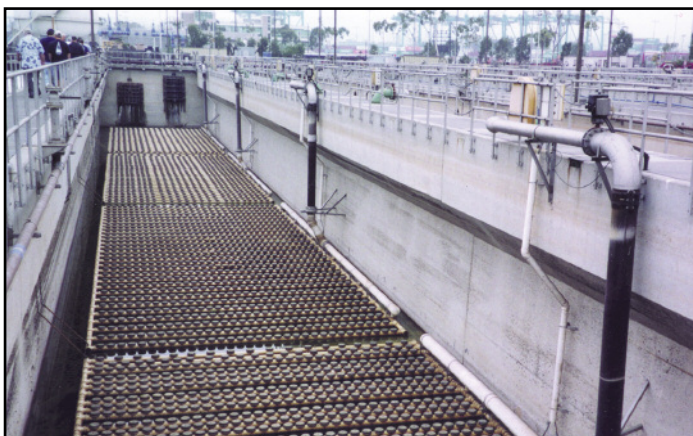
“Bubblers,” shown in this empty aeration tank, pipe in air to stimulate the growth of aerobic bacteria.
