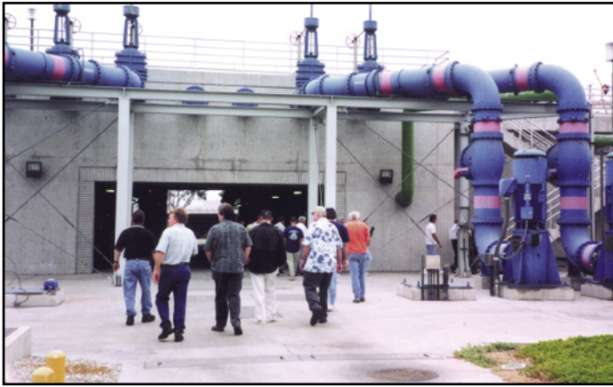
About one third of the clarified liquid goes on for advanced treatment by micro-filtration, starting in this building at the Terminal Island plant.
