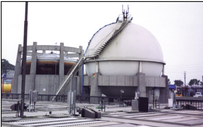
The digestion process produces methane gas, which is piped to these tanks. Some of the methane is used to heat the digesters and some is burned off.
