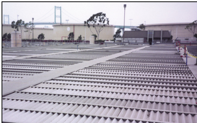
Separation of organic solids from liquids begins in these primary settling tanks.
