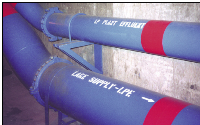
Piping at wastewater treatment plants (process piping) is regulated by ASME. The lower pipe discharges into a recreational lake near the Tillman plant. Note the heavy-duty pipe supports and color coding.
