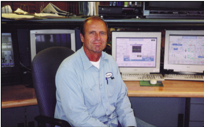
Steve Dapena, Operator 2, in the control room where computers monitor the processes in every area of the Terminal Island Treatment Plant.
