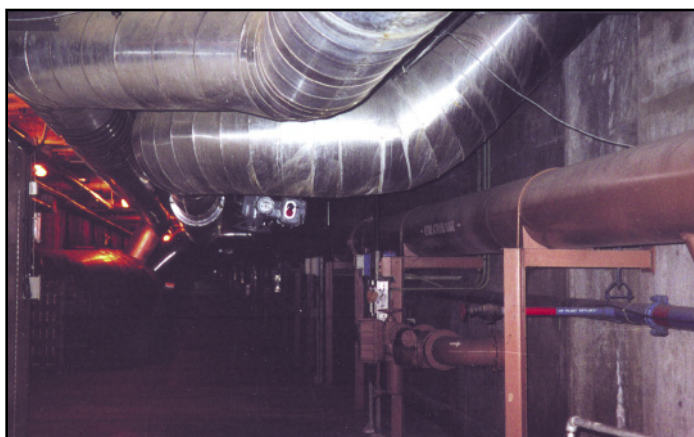
Utility corridor underneath the Tillman plant. The brown pipe transports sludge bound for the Hyperion plant. The overhead air ducts send air to the bubblers in the aeration tanks. Some of Tillman's underground corridors have been used in movies and TV shows for chase scenes.
