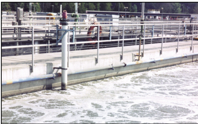
In this aeration tank at the Tillman plant, the remaining organic solids are biologically broken down by aerobic bacteria. Note the life preserver. Kook Dean said nobody has fallen in, but when the tanks are cleaned, they find pagers, wallets and cell phones at the bottom.
