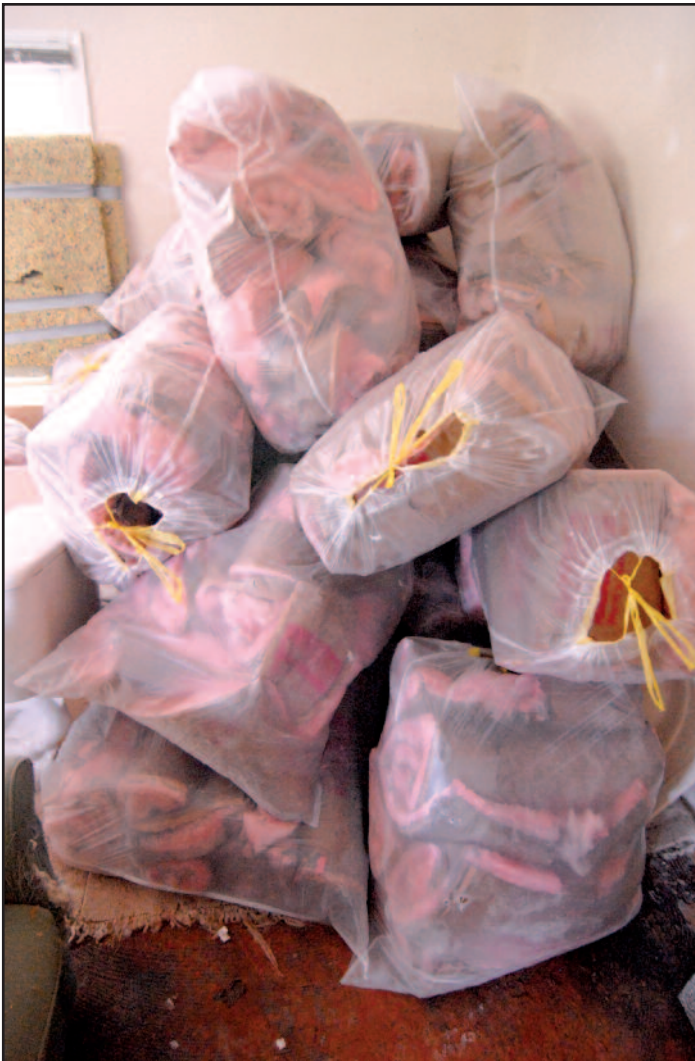
Insulation is recovered and bagged up. Much of it can be recycled and used elsewhere.
