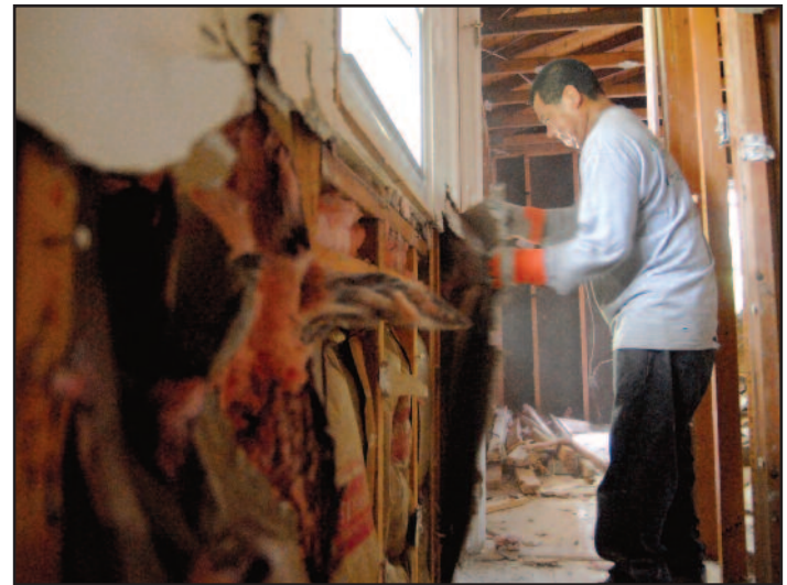
A Deconstruction Services worker carefully removes wallboard and insulation from the home they are deconstructing.
