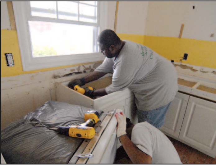
Kitchen cabinetry is carefully disassembled and functioning appliances removed to be resold.
